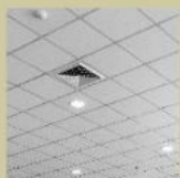
CEILING GRID FALSE CEILING
